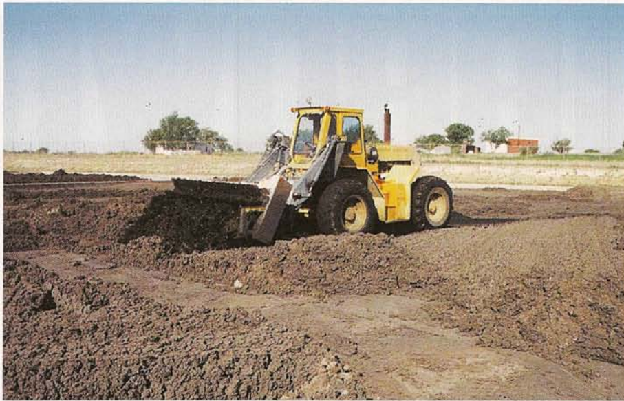
Biosolids ready to be removed from drying beds.
